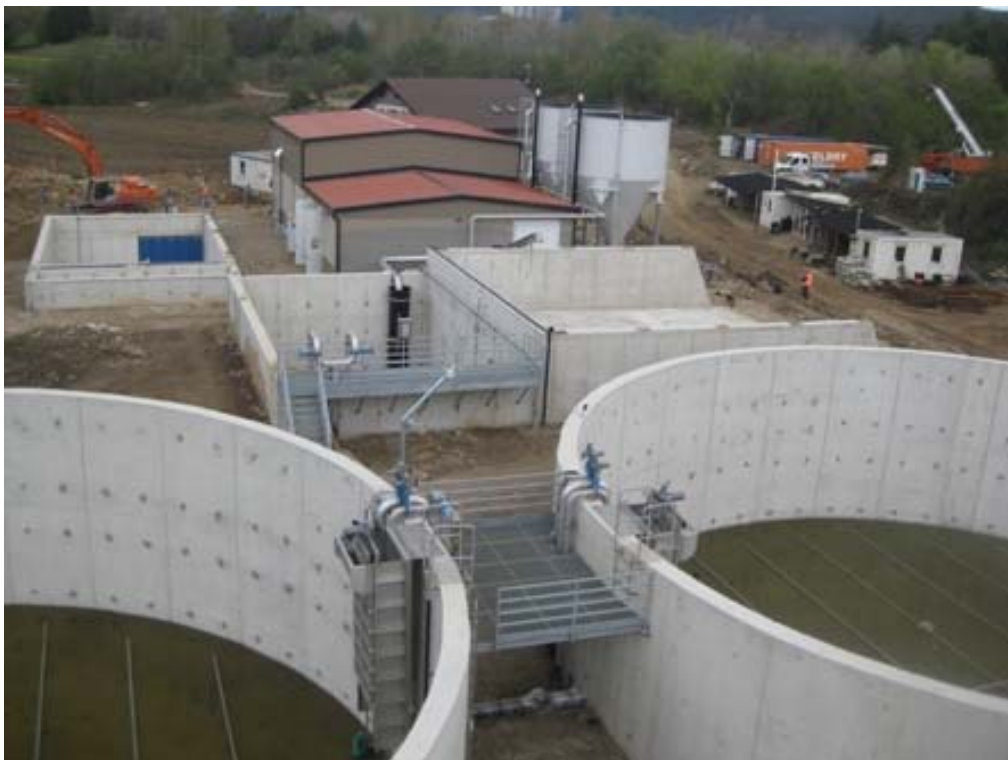
SBR BASINS AND OTHER FACILITIES
